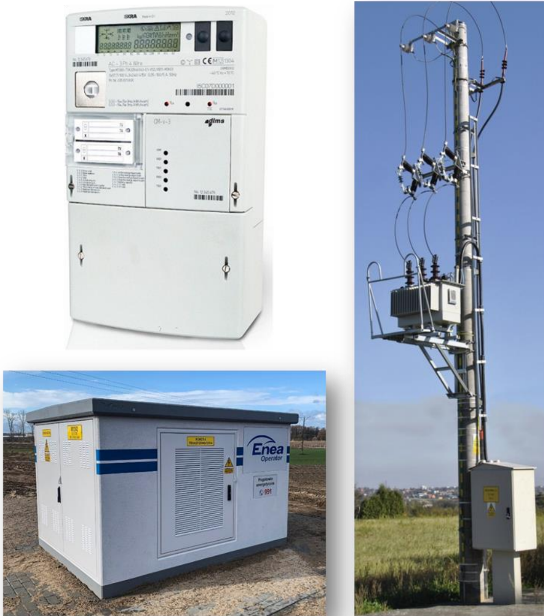
Figure 3. An AMI meter with installation at MV/LV substations
